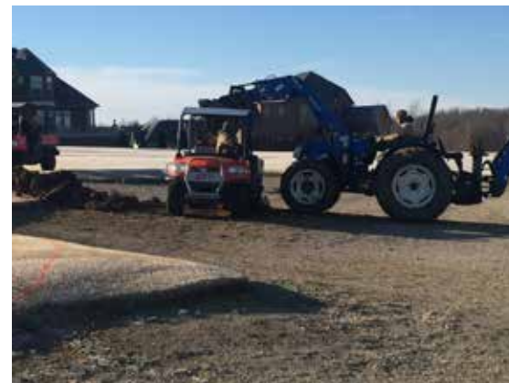
Crews works to remove a protruding "nose" of a target bunker on the range to make it easier to maintain.
