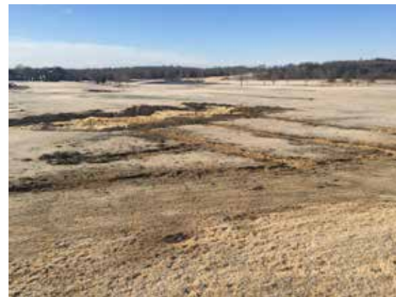
View to the SW from the driving range deck with extensive drainage added.
